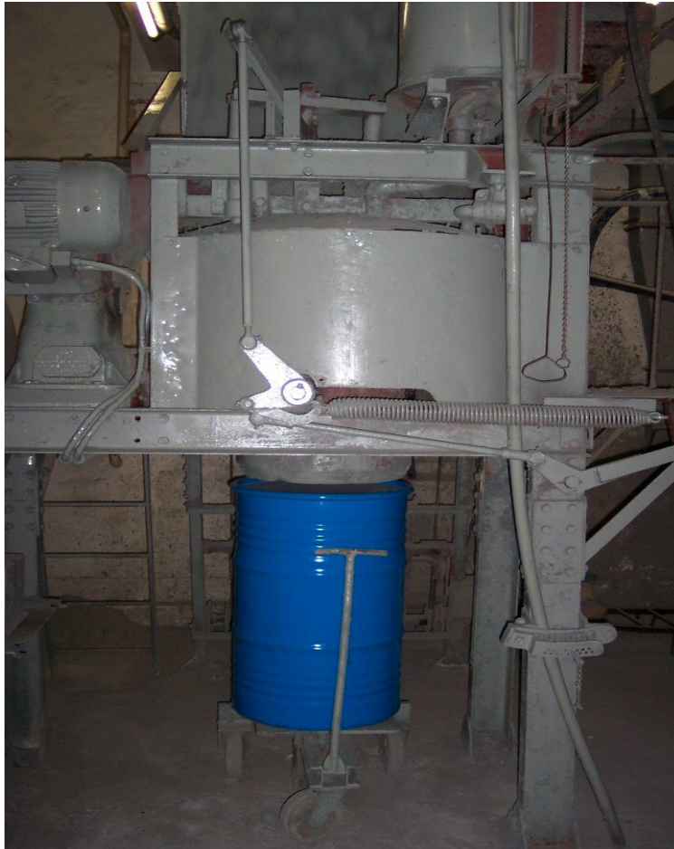
Solid waste cementation installation at STDR Magurele
